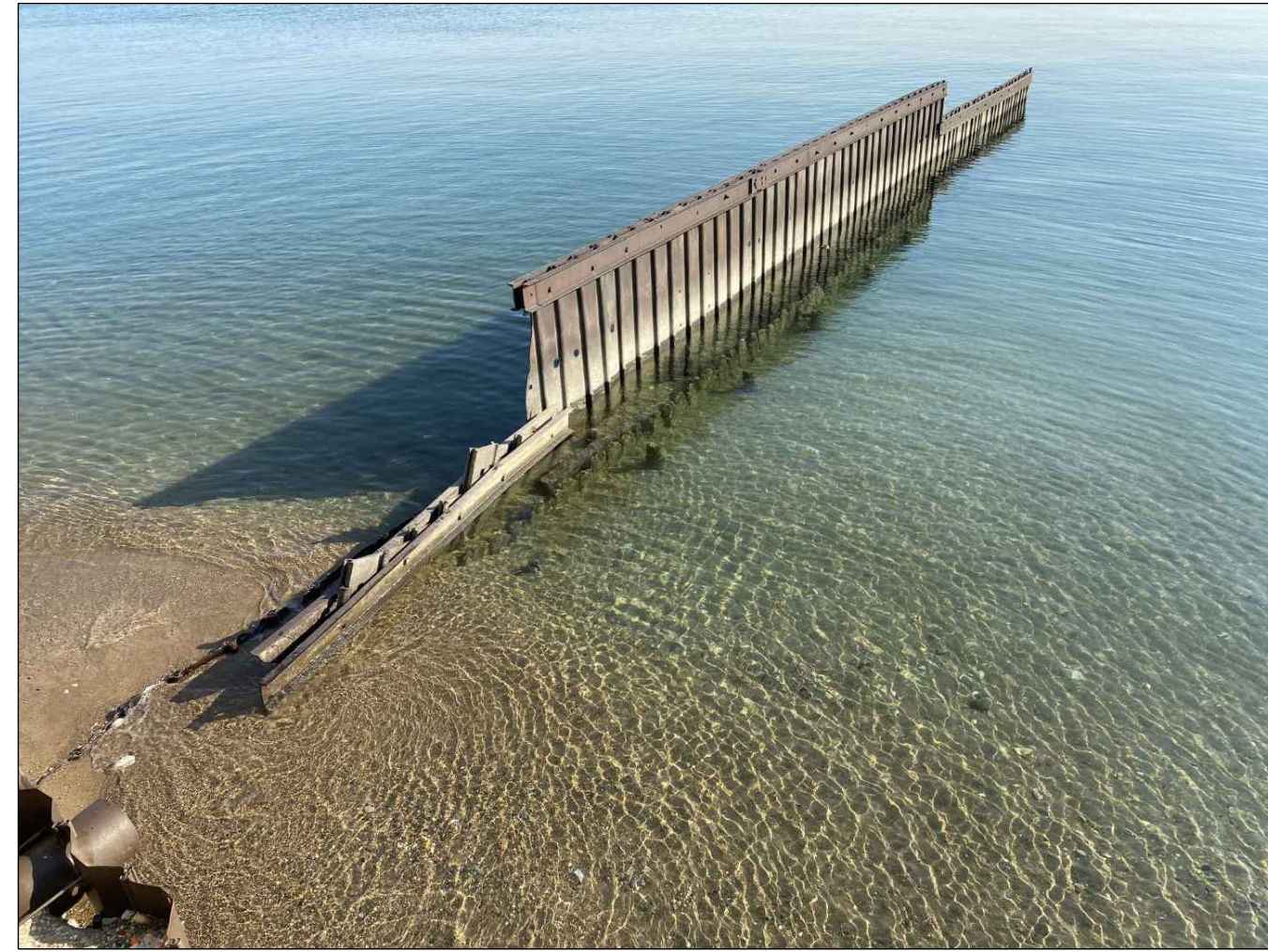
PHOTO 2: LOOKING NORTH AT DAMAGED STEEL SHEET PILE.
