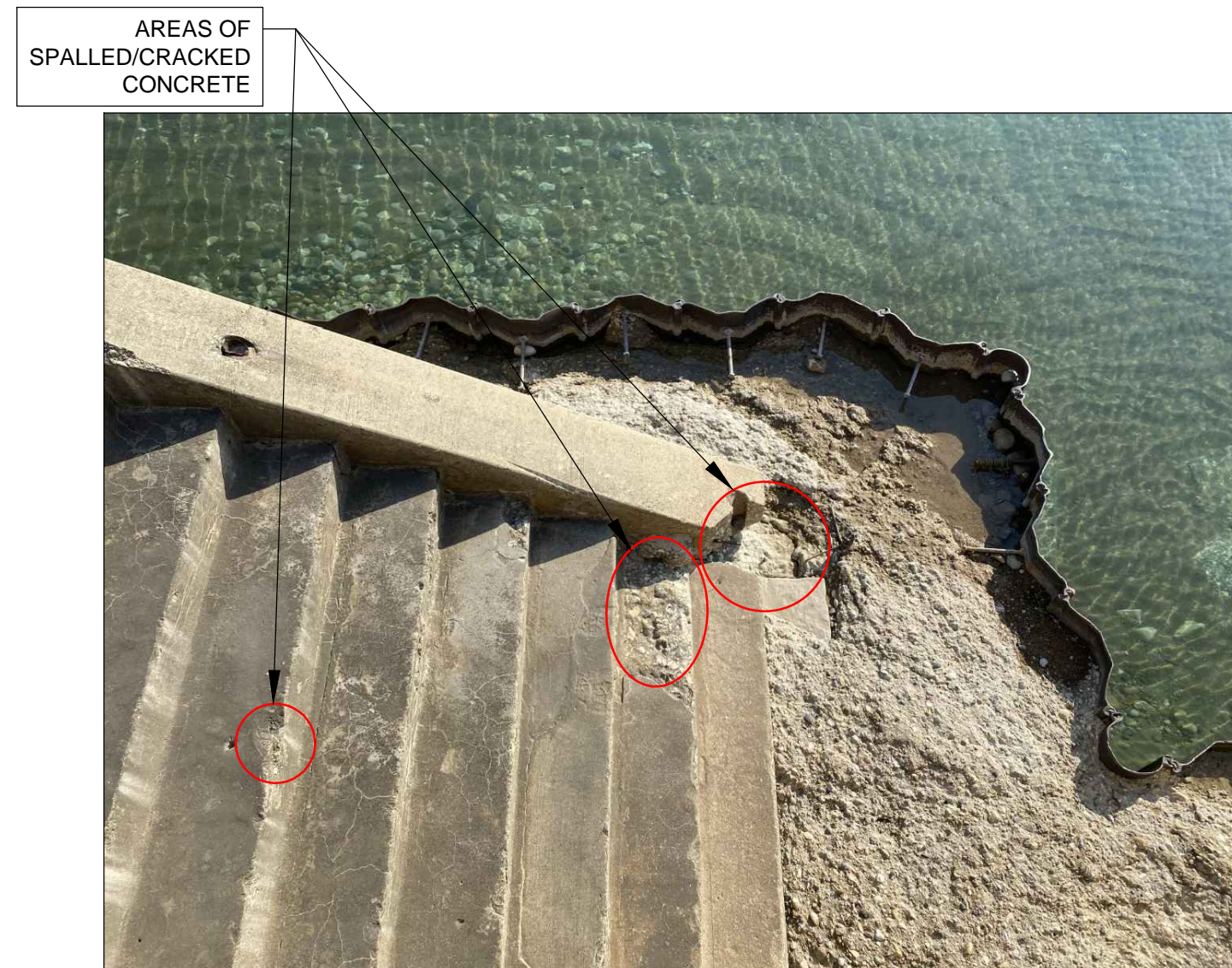
PHOTO 7: LOOKING NORTHEAST AT THE DAMAGED STEEL SHEET PILE CONCRETE CAP AND SPALLED/CRACKED CONCRETE STAIRCASE.
