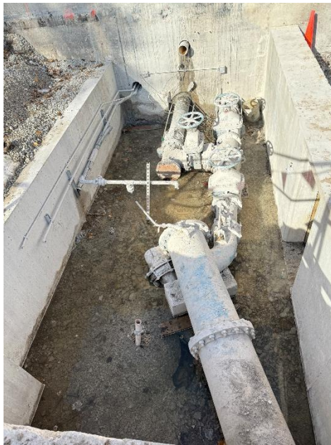
Figure 8: Abandoned water pipes found under the generator room.
