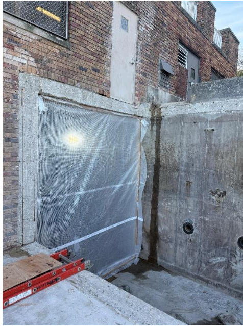
Figure 3: Temporary enclosure of new door entry on the north side of the building.
