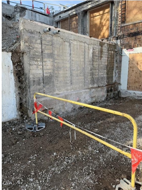
Figure 5: Remaining west wall of the generator room.
