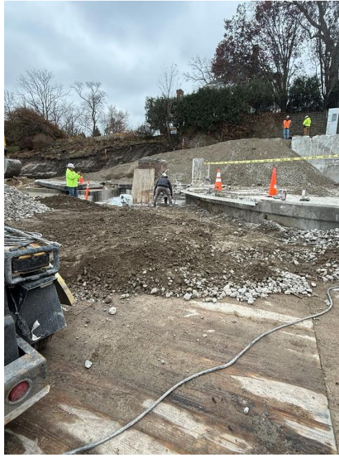
Figure 5: Material placed to allow heavy equipment up the bluff to install the helical piers.
