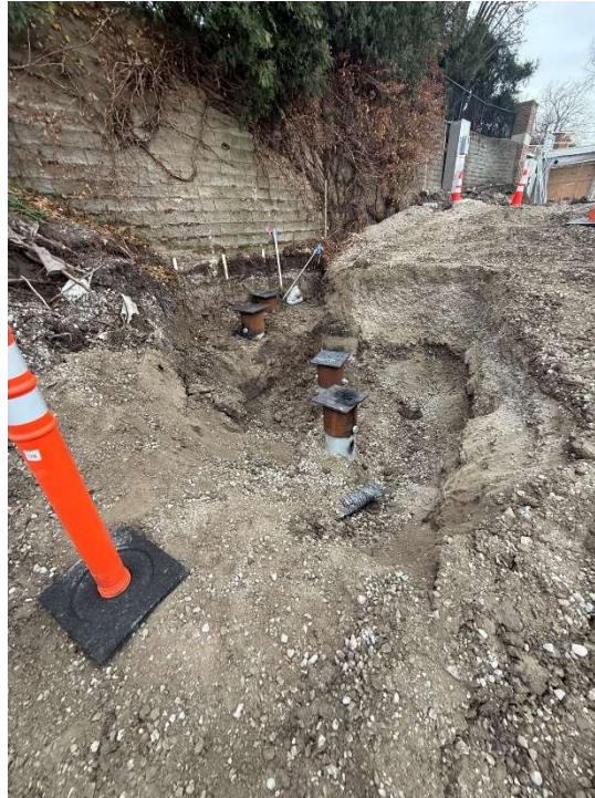
Figure 1: Helical piers cut down the appropriate size to support the concrete and steel for the new ramp.
