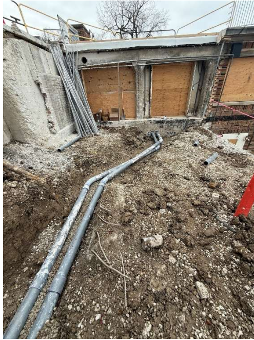
Figure 5: Conduit running from the meter cabinet to inside the building.
