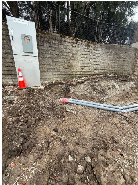
Figure 4: Installation of conduit runs to supply the electrical service to the building and bath house.
