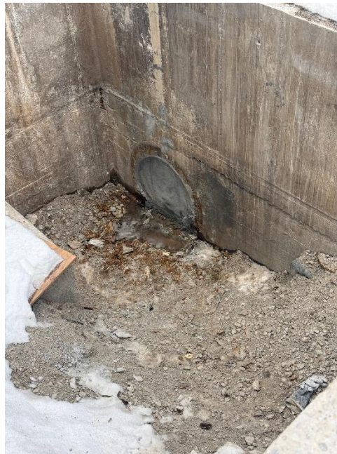
Figure 4: Capping and sealing pipe location to avoid water penetration undermining the new foundation.
