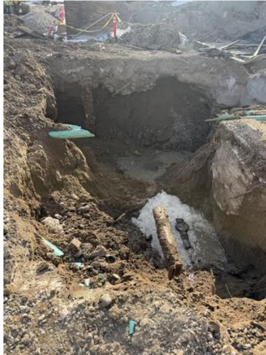
Figure 3: Removal of Unforeseen Underground Obstructions
