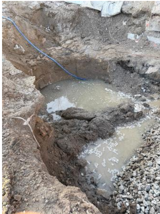
Figure 2: Uncovered Water at Silo
