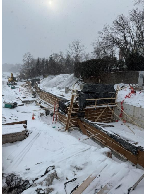
Figure 7: Works working to keep the forms in proper position due to the snow and wind.
