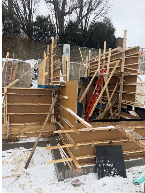
Figure 1: View of the concrete forms being adjusted for electrical and irrigation routes.
