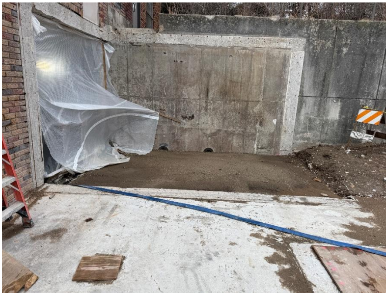
Figure 2: Area on the north side of the building that will have new concrete.
